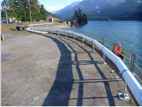
Cascades Island LPS Extension.
